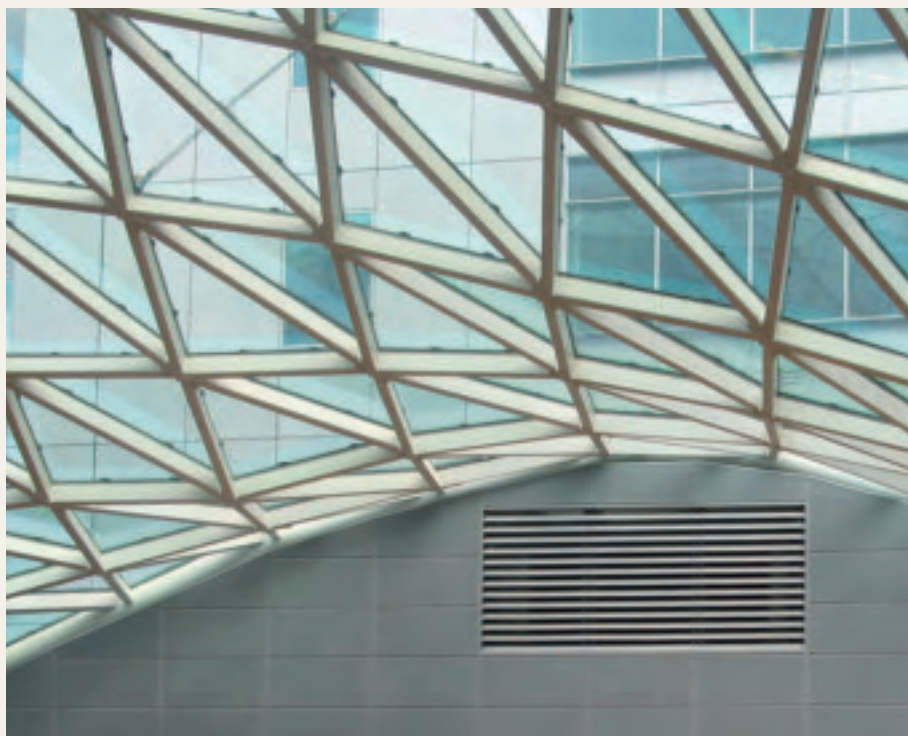
19. Perimeter smoke extract.
