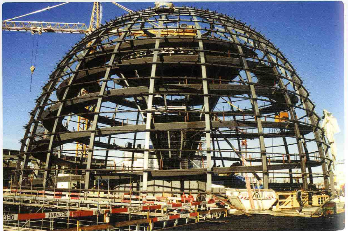
Murphy/Jahn, Sony Center Forum Roof, Berlin, 2000 Previous spread Abseiling for the final installation of the glass panels.
