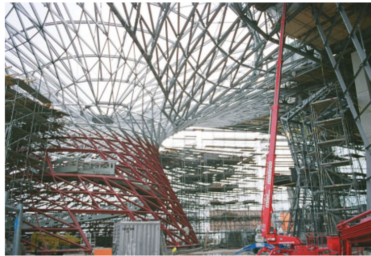
Complex roof structure of the BMW Welt building in Munich by Coop Himmelb(l)au architects and Bollinger + Grohmann structural engineers. See 'Form, Force, Performance: Multi-Parametric Structural Design' on page 20.
