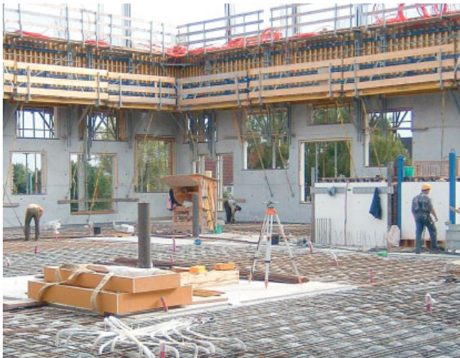
SANAA, School of Management and Design, Essen, Germany, 2006 The void formers and thermal activation pipework in the concrete slabs, as well as the active thermal insulation of hot-water pipes cast into the concrete of the external walls, are still visible during the construction process.
